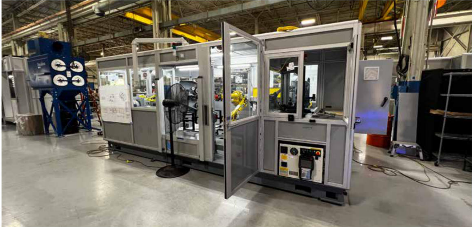
Rotary Turntable System Enclosure
