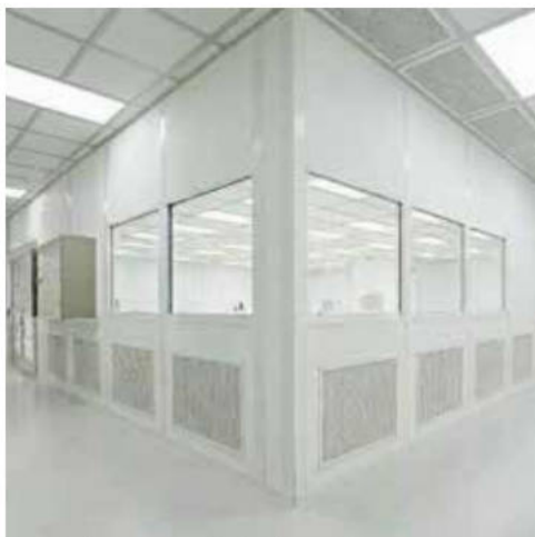
Humidity Controlled Clean Room
