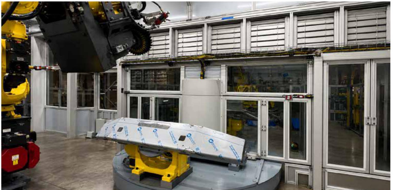
Rotary Turntable System Enclosure
